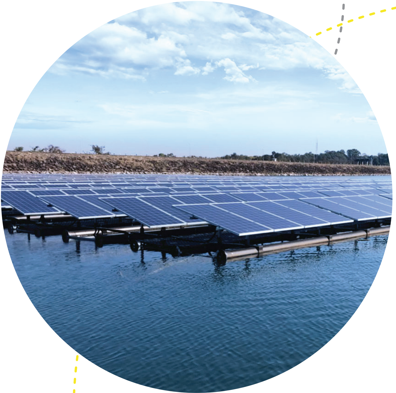
Floating PV system at Sirindhorn Dam, Ubonratchathani Province
