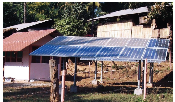
Off-grid PV systems by DEDE
