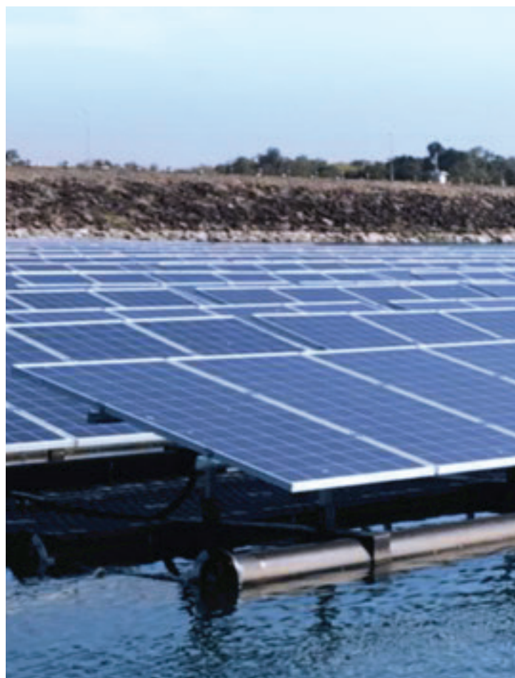
Floating PV system at Sirindhorn Dam, Ubonratchathani Province
