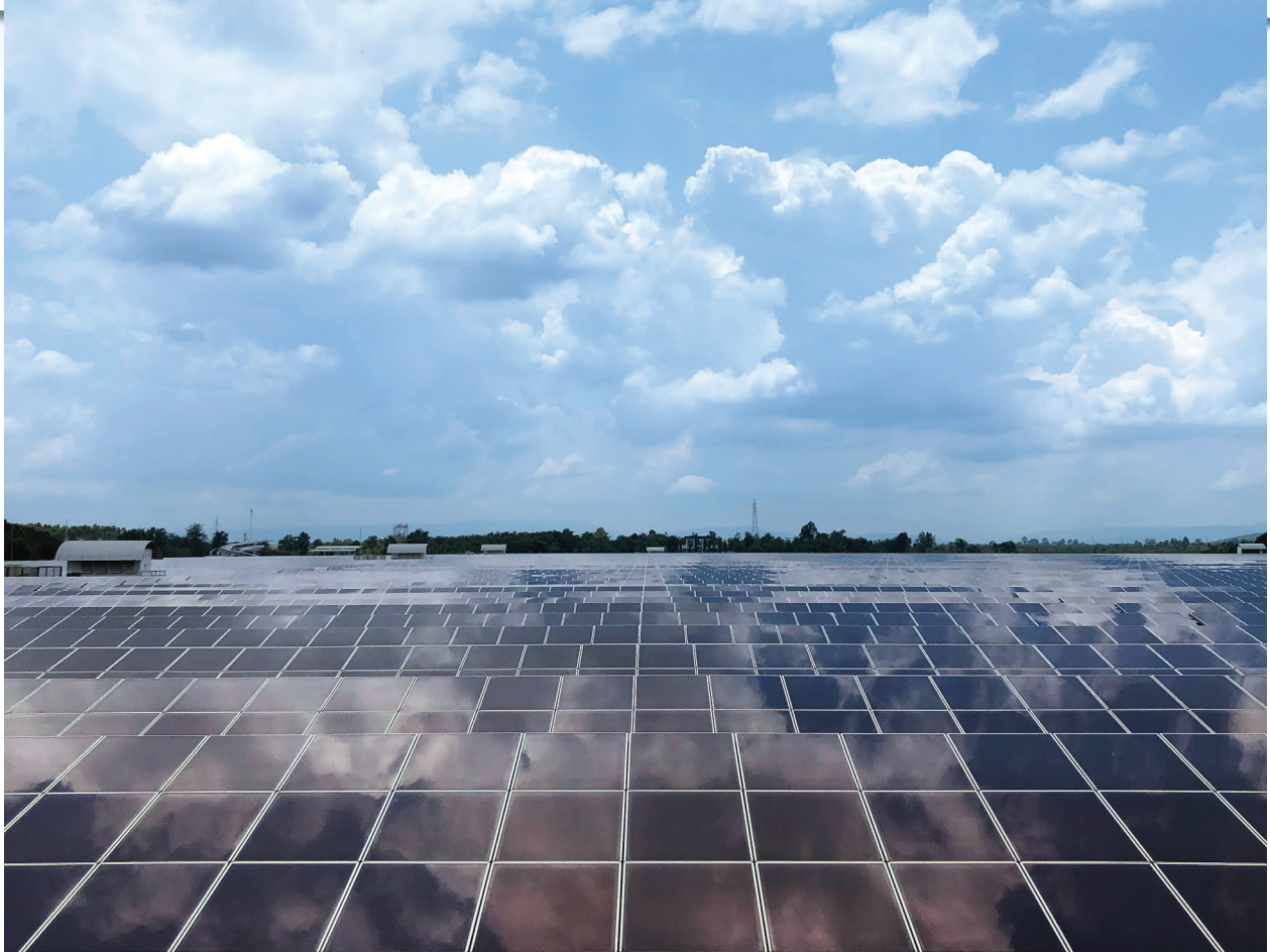
Q Solar1 PV power plant at Kabinburi District, Prachinburi Province
