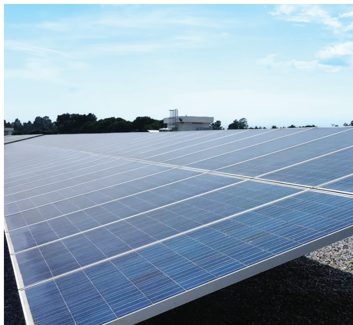
G-Power Source PV power plant at Bung Sam Phan, Phetchabun Province
