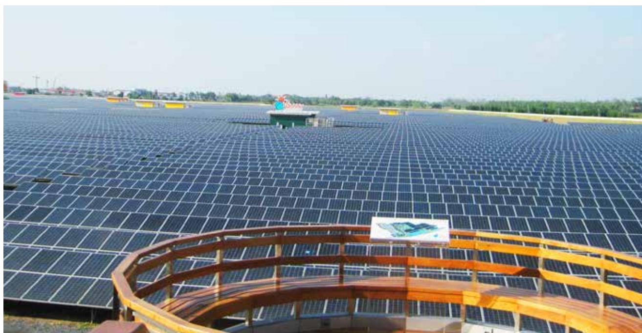
Fig. 2.3 : 35.64 Mwp at Bang Pa-In district, Ayutthaya, which commenced commercial operation in July 2012 (Photo: Bangchak Solar Energy Co., Ltd.)
