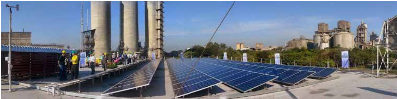
Fig. 2.5 : 49 kWp of PV rooftop system on the business building, at Tha laan district, Saraburi province and operated in June 2014 (Photo: Sci Eco Services Co., Ltd.).
