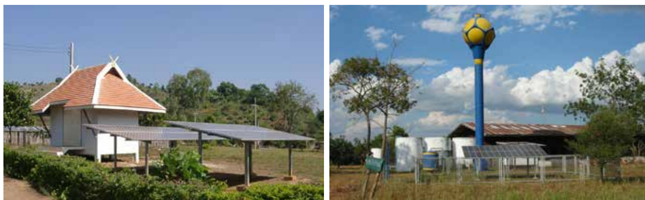
Fig. 2.6 : Stand-alone PV system, (Left) battery charging station at Doi Tung district, Chiang Rai. (Right) PV pumping system at border patrol police school at Phupan, Sakon Nakhorn. (Photo: KMUTT)
